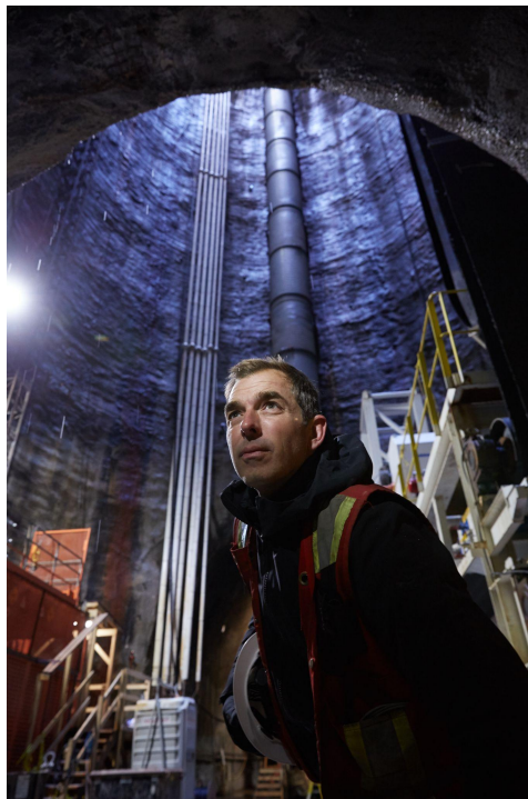
Impossible Repairs' Mike Davidson (pictured), 260 feet below the city of Toronto in the Ashbridge's Bay Treatment Plant Outfall
